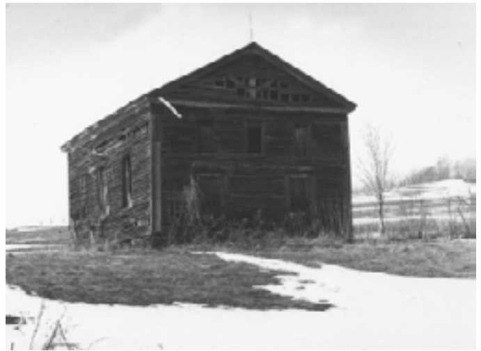
Remains of the East Sullivan Baptist Church on Rt.6, about 8-1/2 miles east of Mansfield. A winter storm brought it down in 1995.
